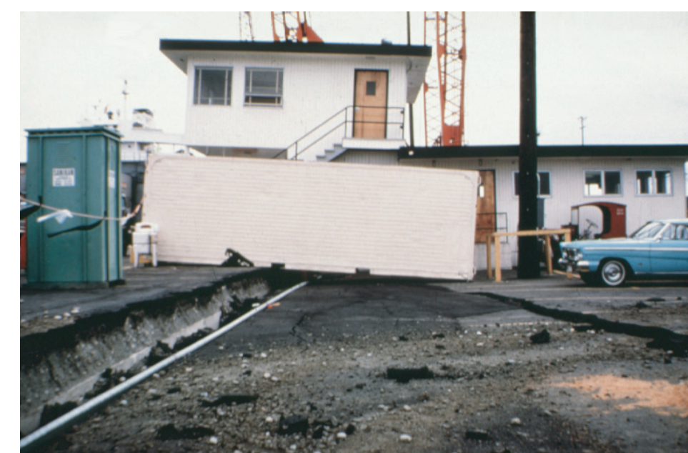
Liquefaction during the 1965 SoTac earthquake caused both lateral and vertical movement of the ground in the Port of Seattle. Cargo cranes such as the one in the background are vulnerable to liquefaction-induced ground displacement. Lateral spreading such as this can cause severe damage to both above-ground structures and underground utilities. Photo courtesy of the Karl V. Steinbrugge Collection, Earthquake Engineering Research Center [ http://misc.berkeley.edu/visual_resources/steinbrugge_collection.html ].
